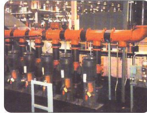
Industrial Plant process piping
